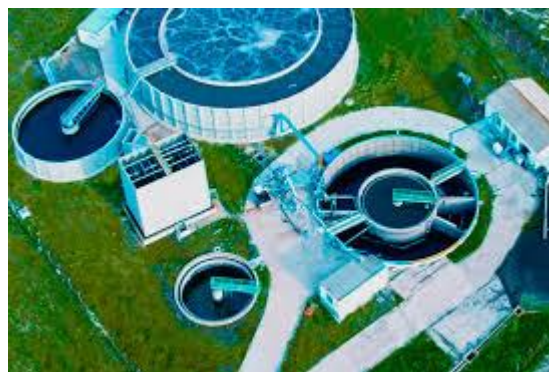
Image 4. Waste water treatment in the textile industry. Source AGUAMBIENTE
